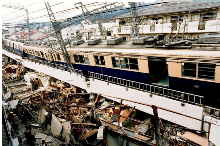
Damaged railway track
