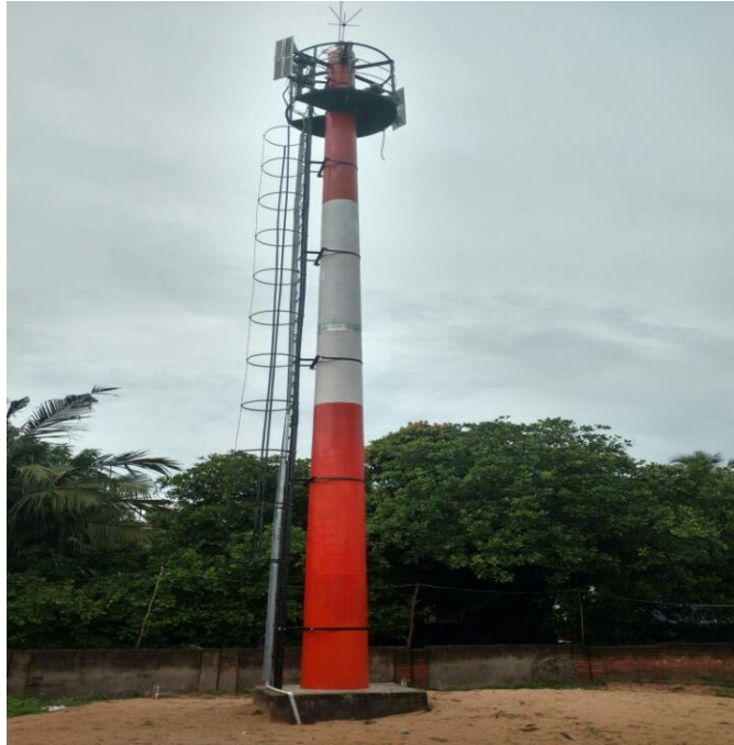
EWDS Spun tower, Ganjam, Odisha
