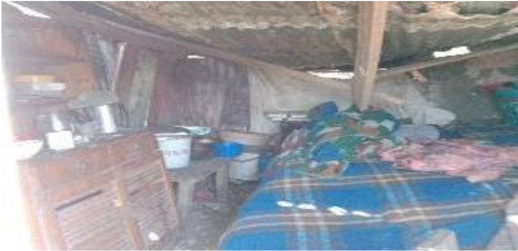
Figure 3: Damaged house in OR Tambo District, EC
