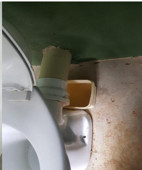
COMMUNITY TRYING MANAGE LEAKING TOILETS IN WARD 2
