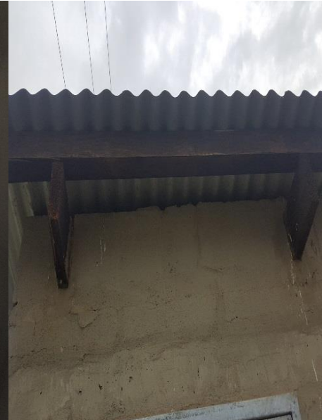
FACILITIES' ROOF AT RISK TO BE BLOWN BY WIND
