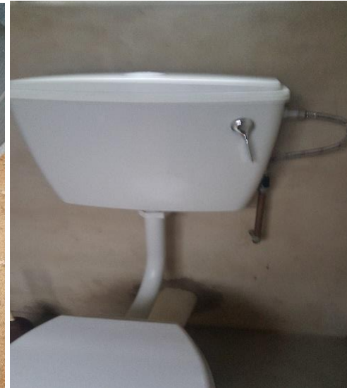
ABLUTION FACILITY FLUSHING HANDLE NOT COMING UP RESULTING TO WASTE OF WATER
