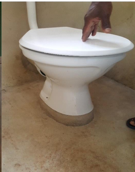
INCORRECTLY INSTALLED TOILET SEAT WHICH LEADS TO WATER LEAKS
