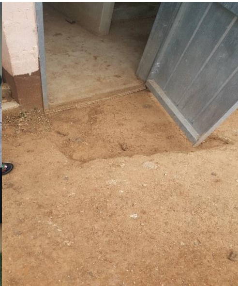
ABLUTION FACILITY FLOODING WHEN IN RAIN
