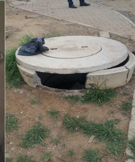
DRAINAGE SYSTEM DAMAGED SINCE IT IS INCORRECTLY INSTALLED ON THE STREET
