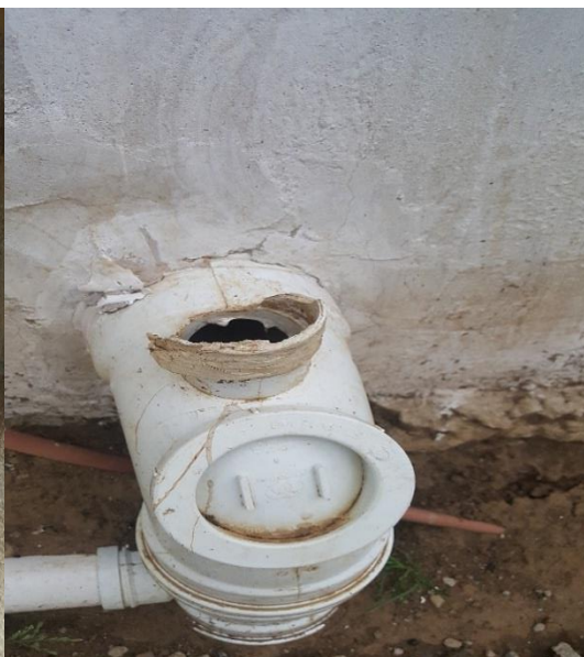
BROKEN DRAINAGE SYSTEM
