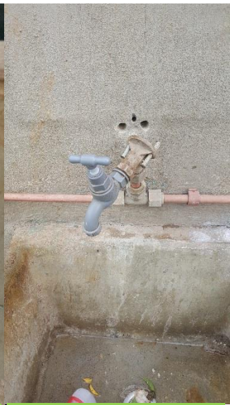
TAP STARTING TO COME OFF DUE TO POOR INSTALLATION
