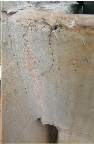
CRACKED CEMENT SINK WHICH WILL EVENTUALLY FALL
