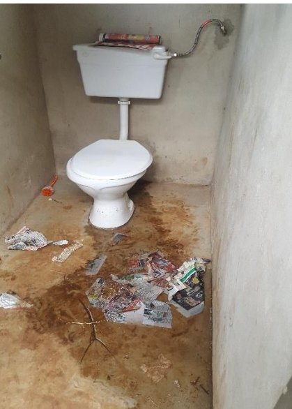
LEAKING TOILETS IN WARD 2
