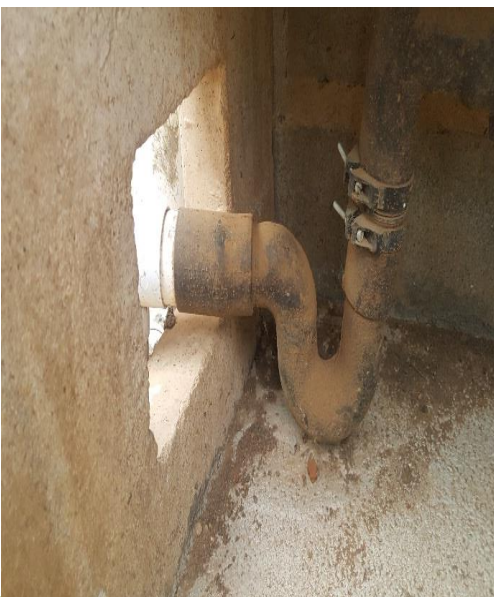
POOR SINK PIPING UNDER THE SINK WHICH RESULTS TO BLOCKAGES
