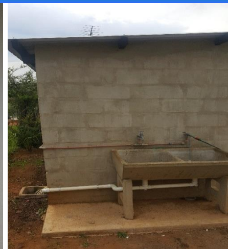
OUTSIDE SINK AND ITS PLUMBING
