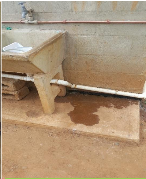
POOR PLUMBING RESULTING TO WATER LEAKS
