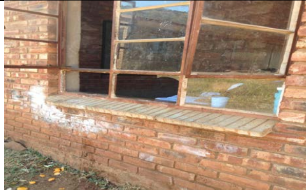
Figure : Broken windows in classroom at Mpandeli Secondary School, 2015
