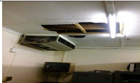
Figure : Damaged ceiling in office at Toekomsrus MCCC, 2015
