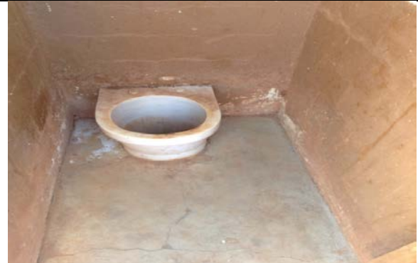
Figure : Broken, filthy learner toilet at Mpandeli Secondary School, 2015
