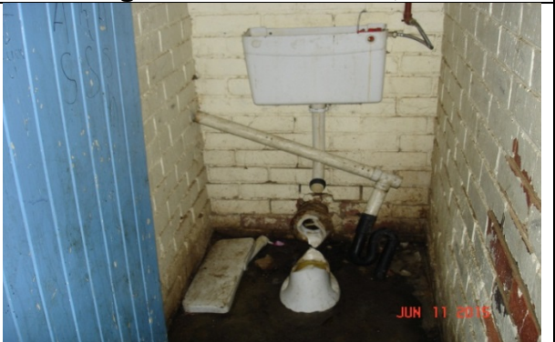
Figure : Broken, dirty learner toilet at Polokong Combined School, 2015
