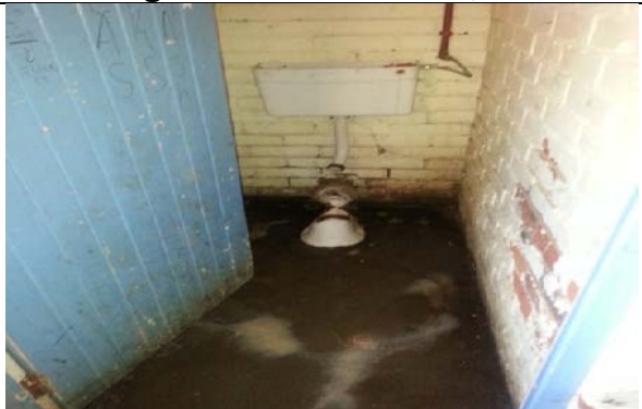
Figure : Broken, dirty learner toilet at Polokong Combined School, 2014
