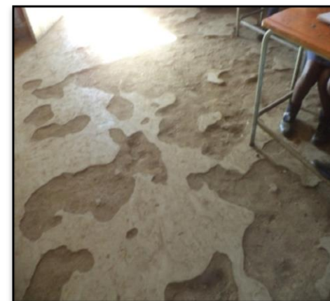
Siwali Junior Secondary School (EC): 'pothole' floors
